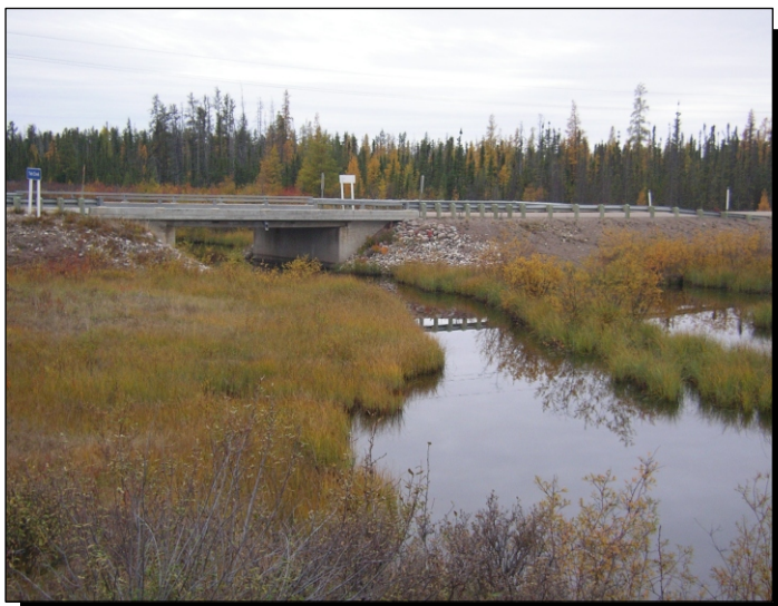
Photo 27 Twin Creek Station 1 and Water Station 11.
