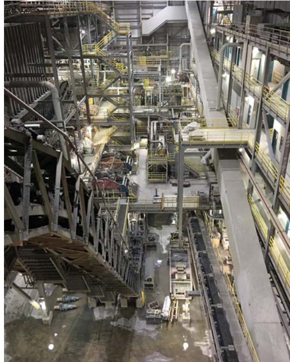
Inside the plant. Note the large covered square pipe on the right where mined rock enters the plant.
