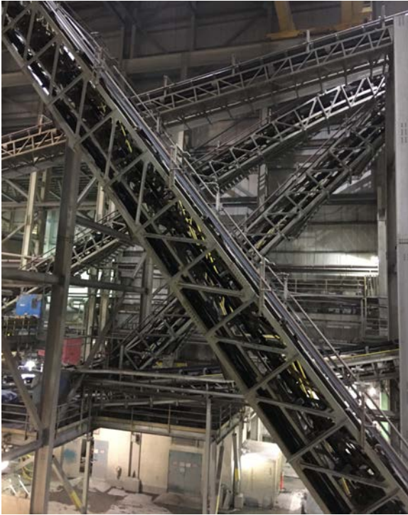
Conveyor belts move crushed rock.
