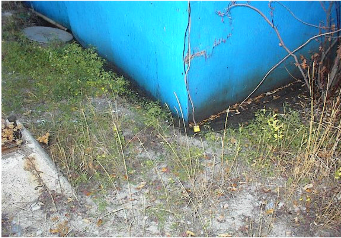
Photo 19: Minor oil staining around gear house on southern landing.
