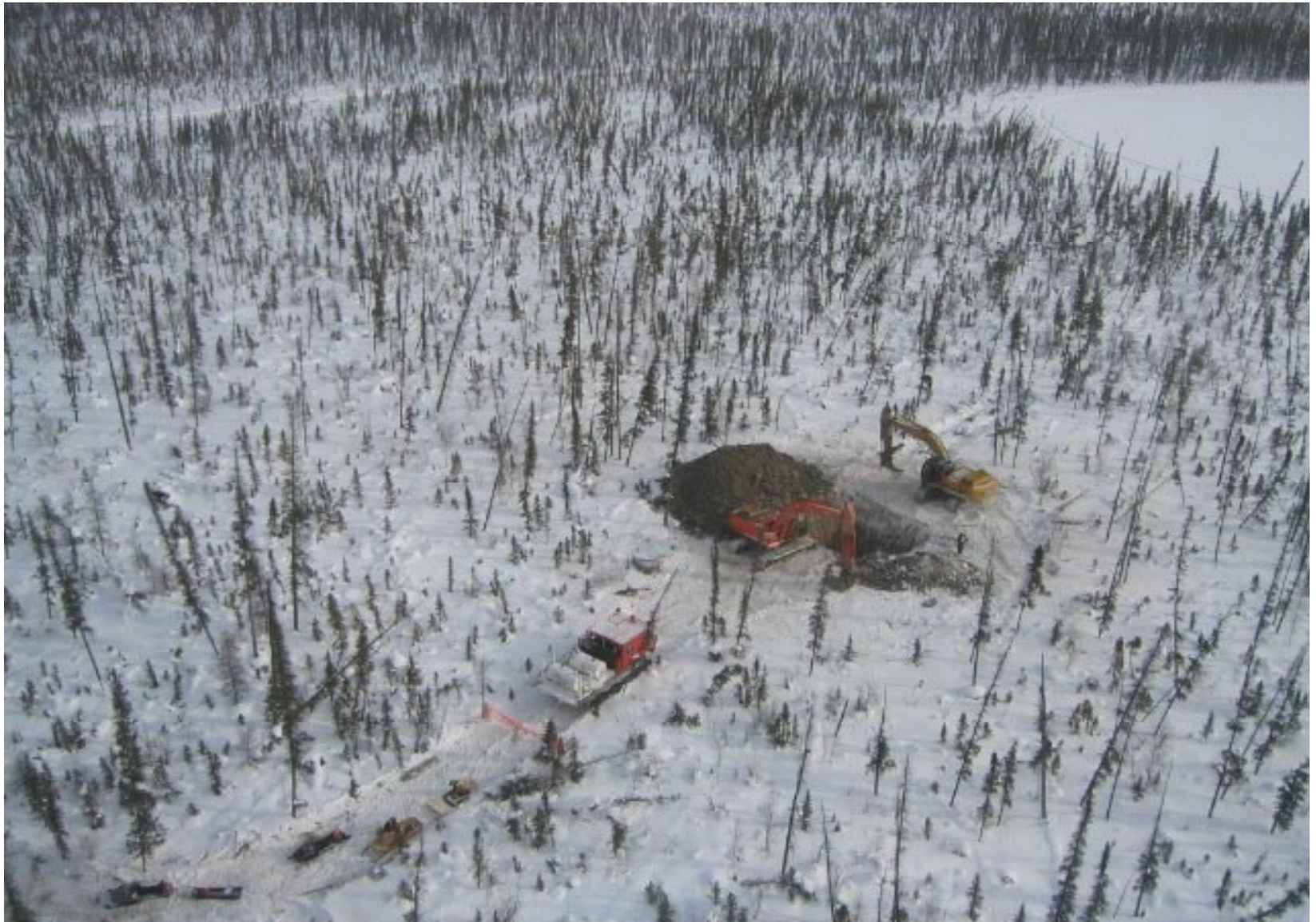
Operations: Excavating test pit at Site 6.042P in Sahtu K'ahsho Got'ine Winter 2004
