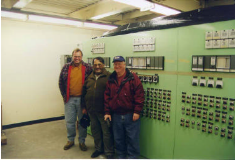
Mill Control Room
