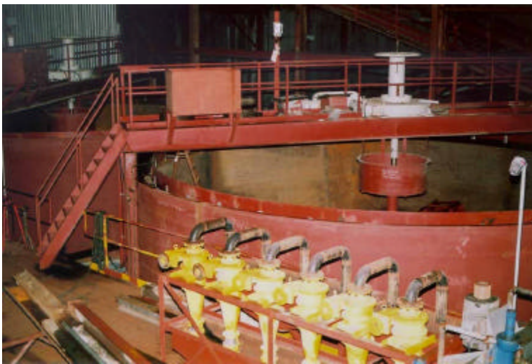
35' Thickener with Tailings Cyclones in Fore Ground
