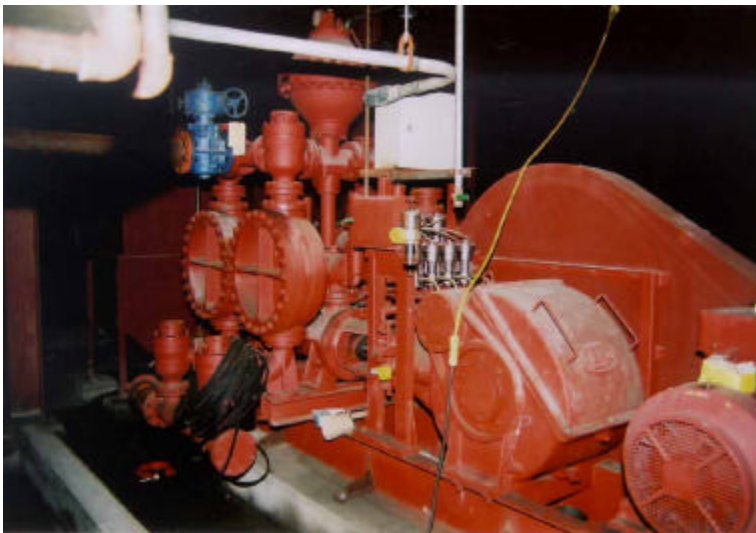
Geho Pump (Mill Basement)
