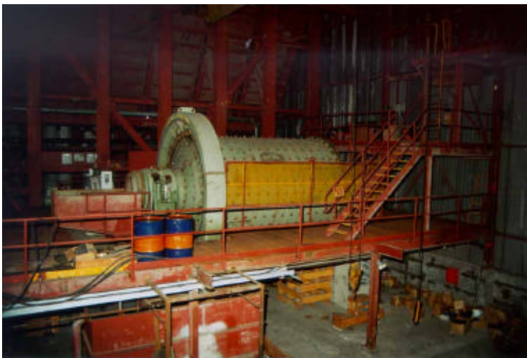
Ball Mill, View from Mill Control Room
