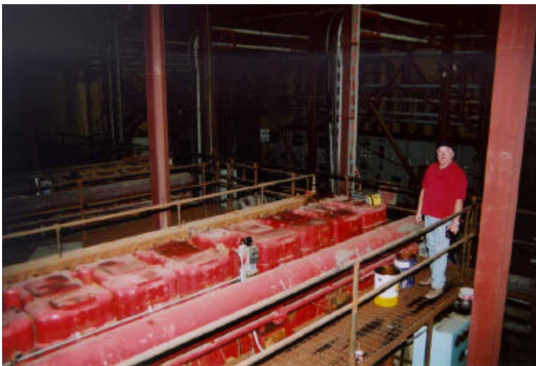
1150 HP Cooper Bessiner Unit (1 of 4)
