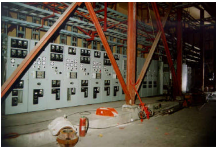
Power house – Motor Control Center
