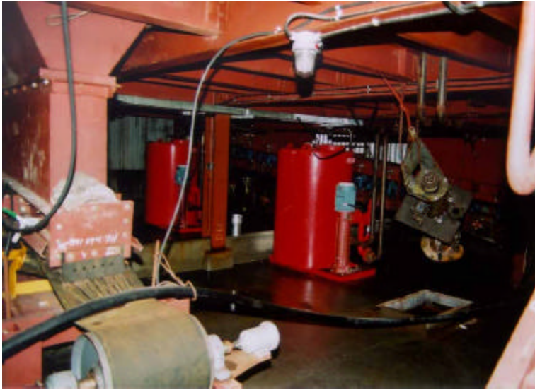
Larox Pressure Units ( Mill Basement)
