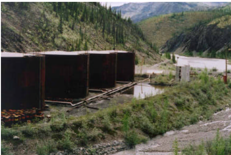
Fuel Tank Farm
