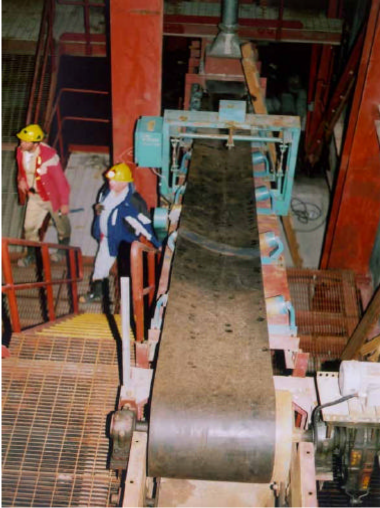
Metal Detector & Conveyor (Crushing Plant)
