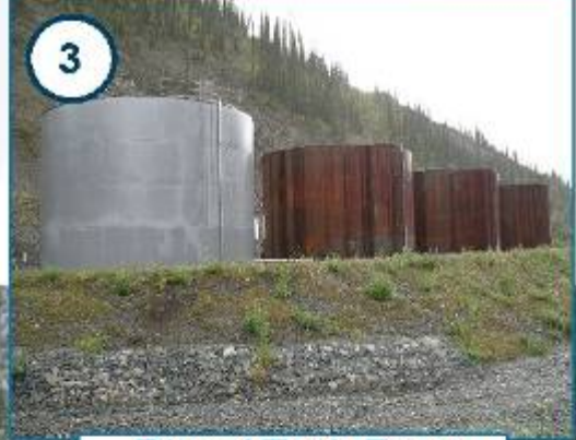
Diesel Tank Farm
