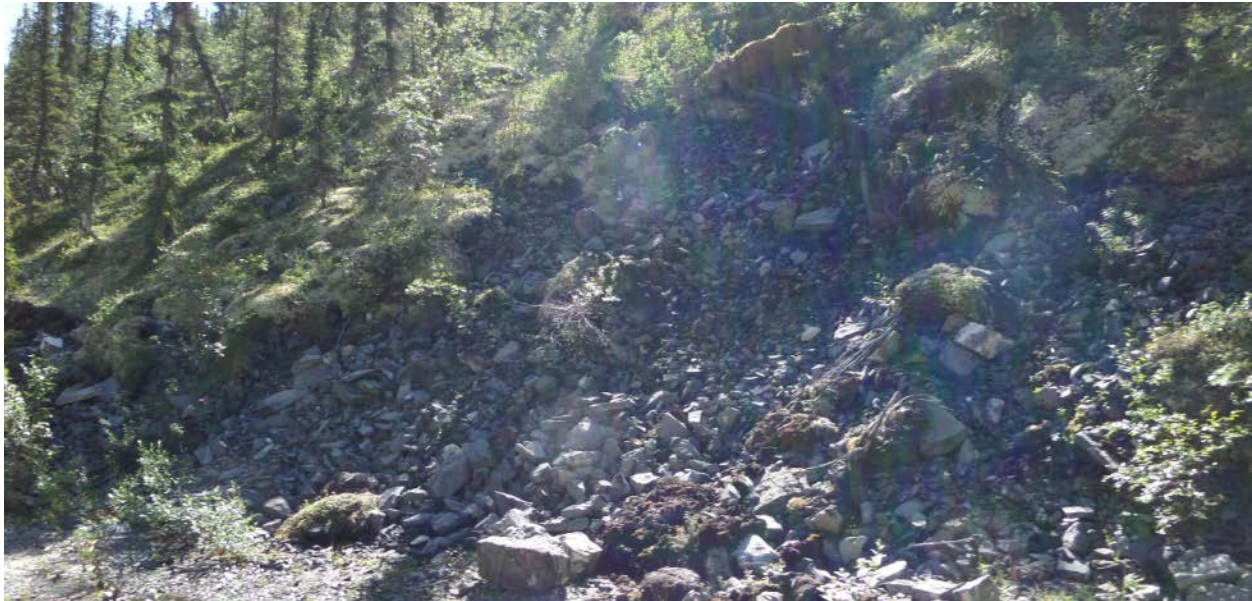
Figure 12-1: Permafrost thaw or creep in borrow pit #10 (PR#62 p6)
